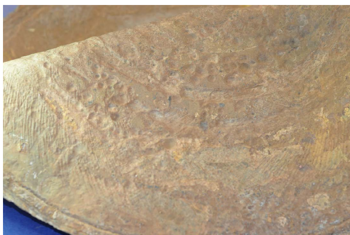
Figure 9. Interior “surface of the moon” condition of the tank circle that separated from the SCR vessel during its catastrophic failure on April 3, 2017. The tank circle was installed in 2012
