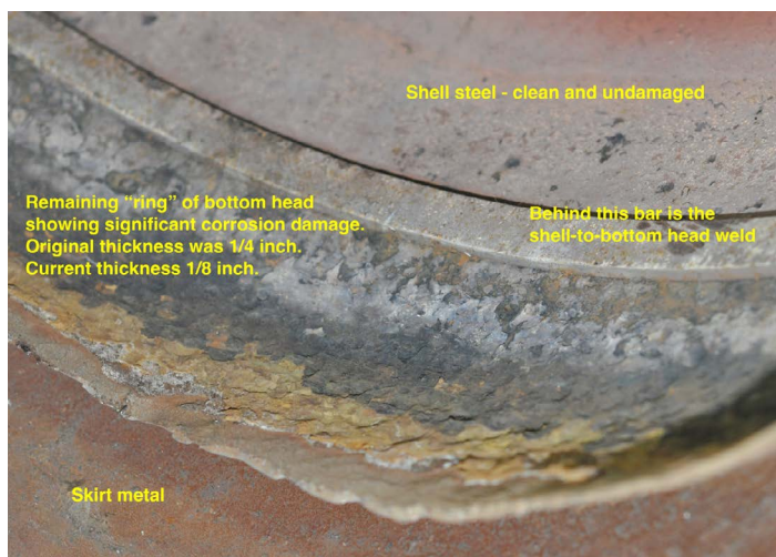
Figure 6. Photo showing 3-4" highly damaged section of the original bottom head remaining in SCR
