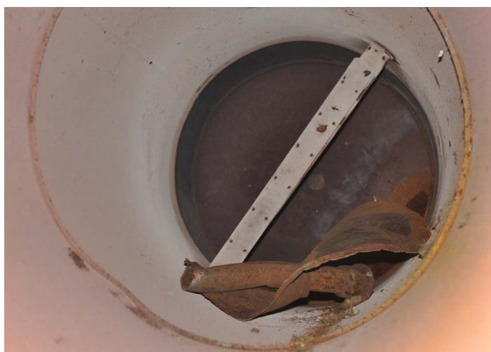
Figure 10. Piece of bottom drain piping and a section of the bottom head
